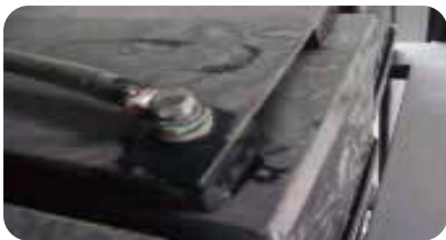
Terminal acid leakage
