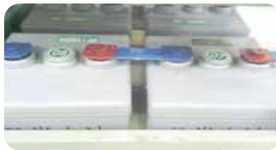
Leakage from battery cover
