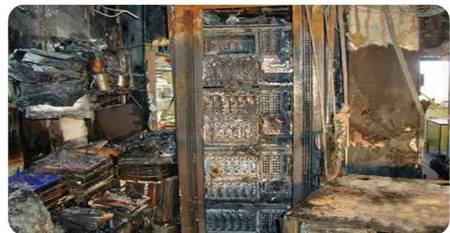
Significant operational and financial losses
